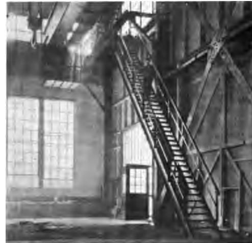
Fig. 6. Stairway and Platform for Crane.*
